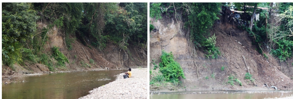
Gambar (Figure) 4. Kondisi longsor di kawasan sempadan sungai ( Landslide conditions in river boundary areas )
